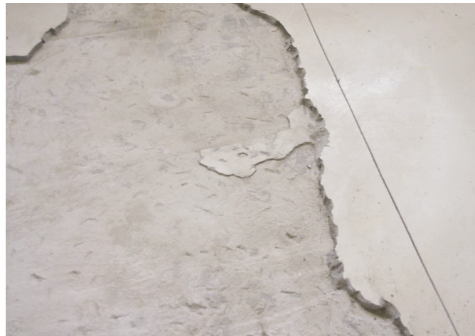
Photo 3. Cracks and loosening of the screed layer of too small thickness
