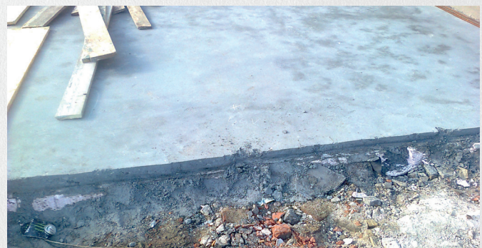
Photo 2. Tarnish on the surface of a floor screed
