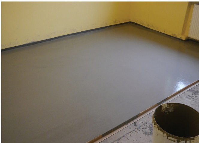
Photo 2. The intermediate expansion joints determine the technological areas in the shape of a square or similar.
