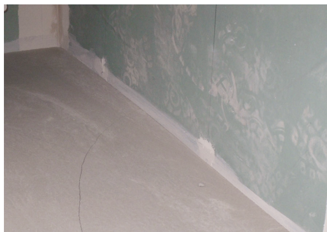
Photo 5. Shrinkage cracks of the screed. No peripheral expansion joints along the walls
