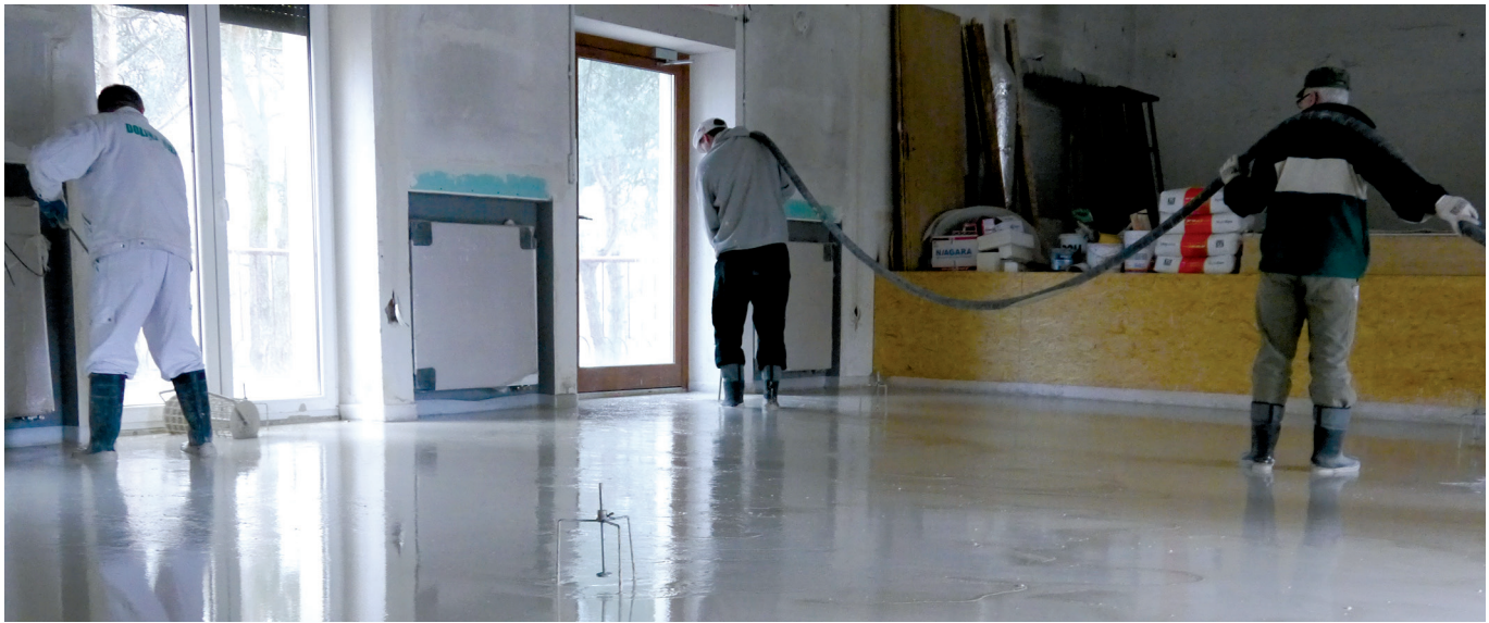
Photo 2. Machine application of the fast-setting anhydrite-based screeds is a perfect solution for large surfaces (over 15m 2 )
