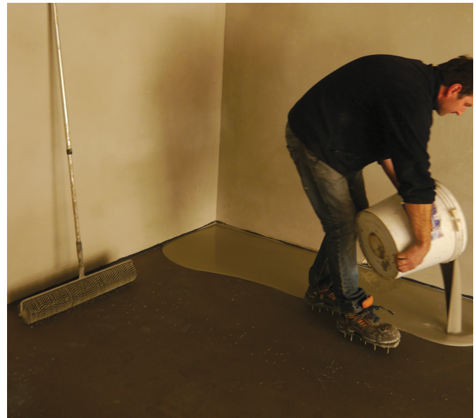
Photo 3. The mortar should be poured in even layers; one should commence the application from the wall which is the furthest from the entrance.
