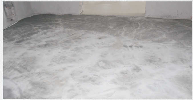
Photo 1. Tarnish on the surface of a floor screed
