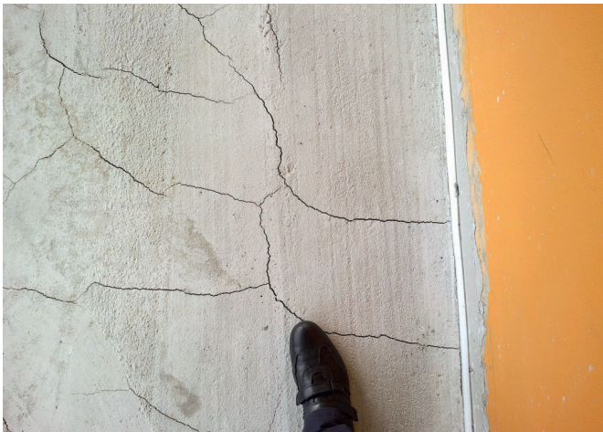
Photo 6. Cracks of the substrate
