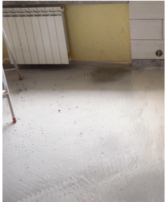
Photo 8. Addition of insufficient amount of water results in difficulties in smoothing the surface finish
