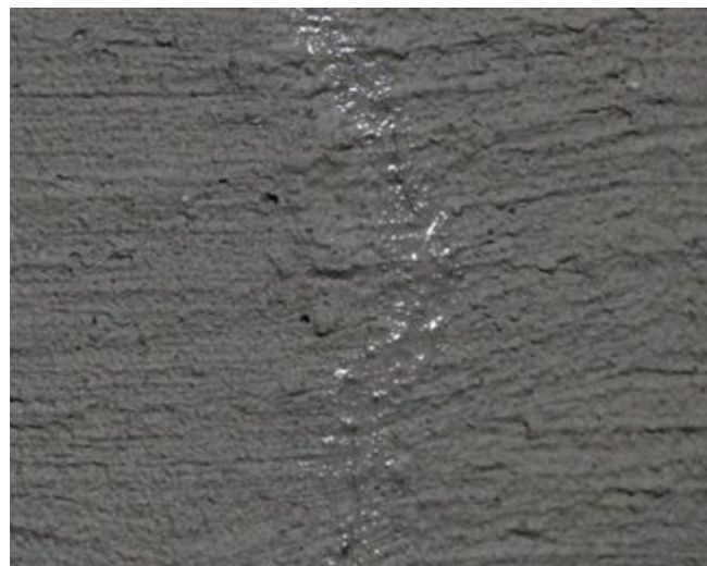
Fig. 3. Gradual closing of the crack by crystallising salts, minor water seepage still present. Effect after 7 days.
