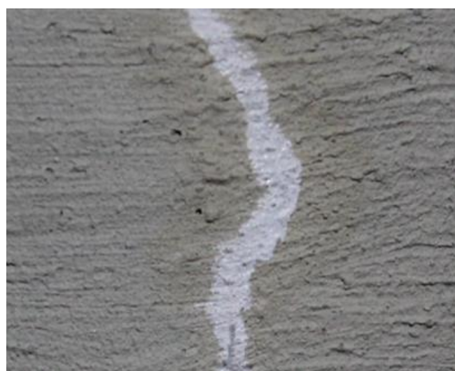
Photo 4. Closure of the crack by salt crystals, no oozing. Effect after 21 days.
